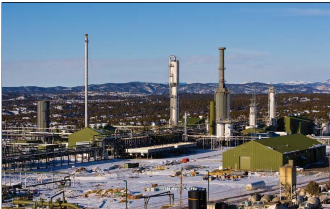
Enterprise Products Partners LP in March 2009 began operations at its Meeker II natural gas processing plant in Colorado's Piceance basin. The Meeker II expansion doubles processing capacity at the complex to 1.5 bcf/d with the capability to extract as much as 70,000 b/d of NGL. Inlet volumes at Meeker at start-up were 750 MMcfd, with 38,000 b/d of NGL being extracted. The company predicted gas volumes to reach 1.1 bcf/d by yearend 2009, when NGL production would reach 60,000 b/d. Photo from Enterprise Products.
