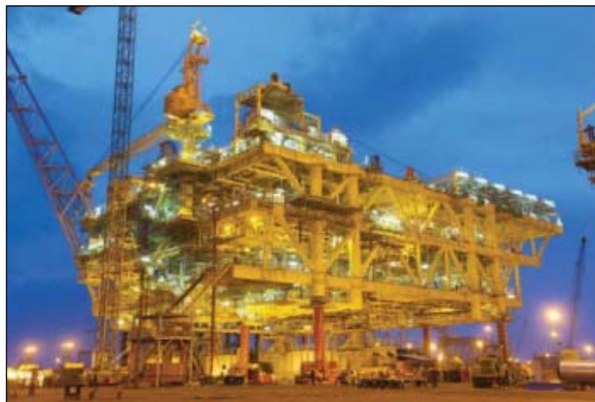
The construction contractor completed all deck fabrication and precommissioning activities on the 15,150-tonne CPP deck before its sail-away from Batam in August 2008 (Fig. 3).
