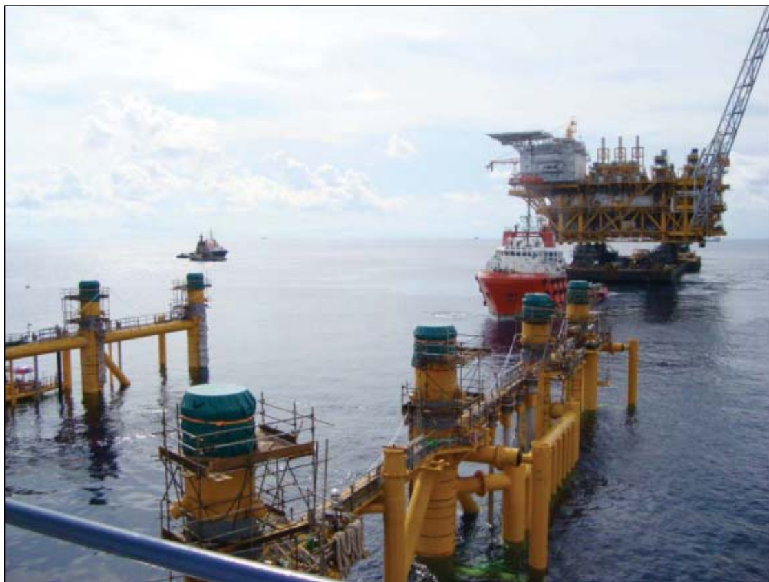
A float-over operation in September 2008 placed the CPP deck on top of the jacket (Fig. 4).
